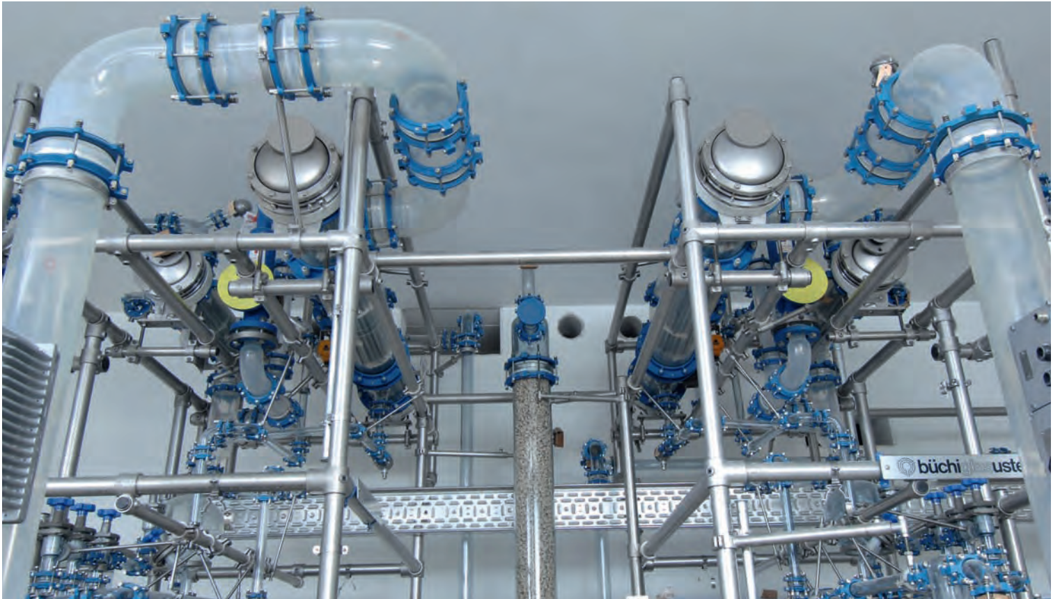
Distillation overhead with SiC shell and tube heat exchangers
