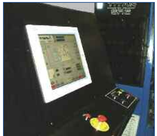
Titan SR6 control desk - upgraded
