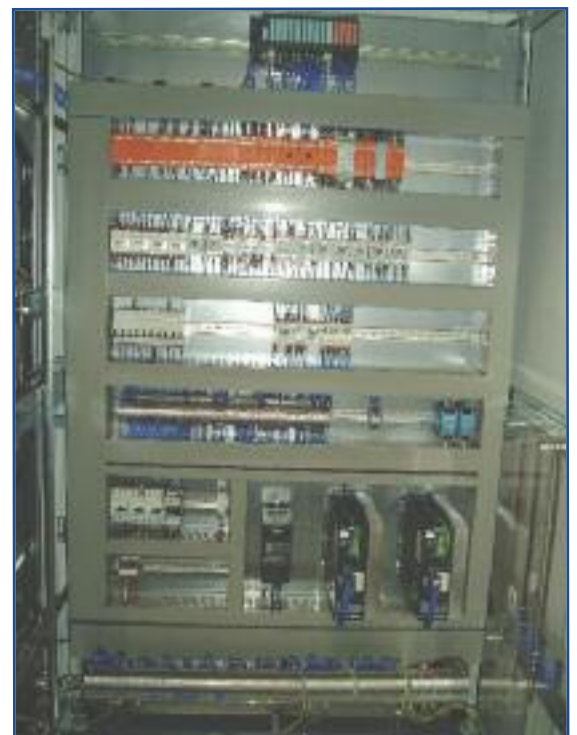
Upgraded machine control panel
