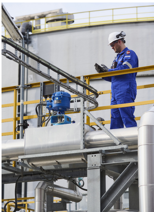
Figure 4. A CVA process control actuator being inspected by a Rotork engineer.
