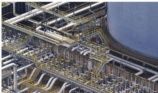
Figure 2. A large number of electric IQ intelligent actuators installed at a tank farm.
