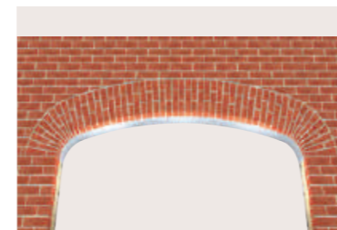
View showing the underside of IG's Parabolic Arch BSFL. This illustrates how the brickwork returns under the soffit of the lintel to ensure no steelwork is visible on the outer leaf.
