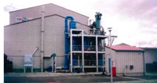
Flue gas treatment for precious metal recovery smelter, Japan
