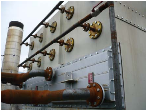
Drawer-type Heat Exchanger Cooler below Pre-Filter Irrigation Spray Bar Connections
