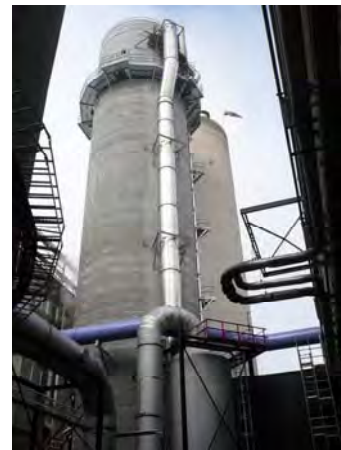
Ground level Candle Filter Vessel after Prilling Tower
