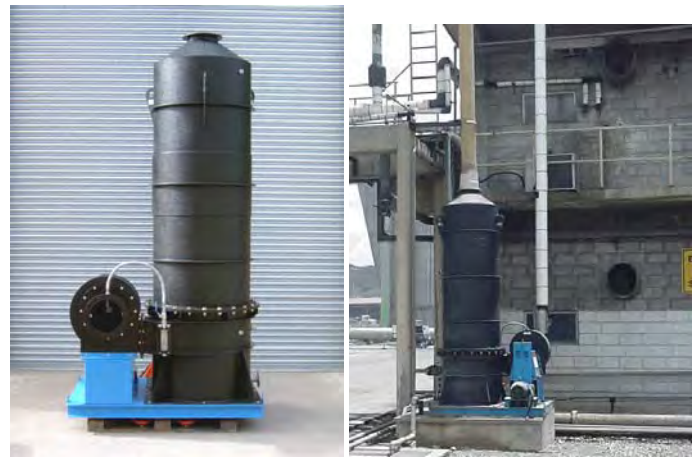
Becoflex BFCF unit on Oleum tanker loading duty
