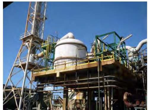
Wet Catalysis Plant filter vessel
