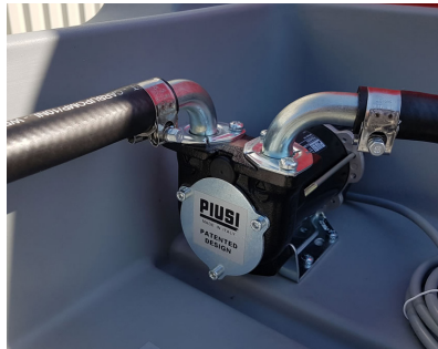
FUEL DISPENSING PUMP
