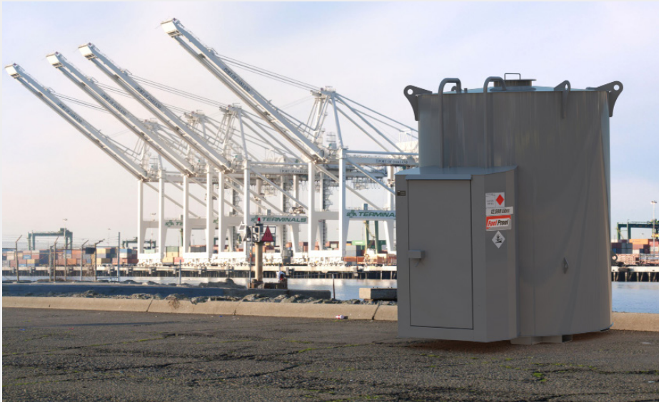
12,500 LITRE VERTICAL BULK DIESEL TANK
