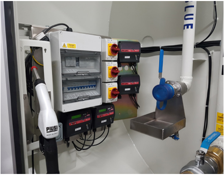
DISPENSING EQUIPMENT, ADBLUE FILL POINT AND DISTRIBUTION BOARD
