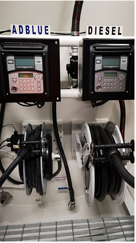
DIESEL/ADBLUE DISPENSING SYSTEMS
