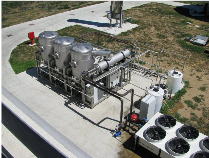
Triple effect evaporator with dry cooler
