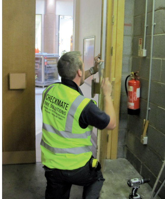
Building occupiers can tailor their maintenance regimes to the criticality and usage of each door
