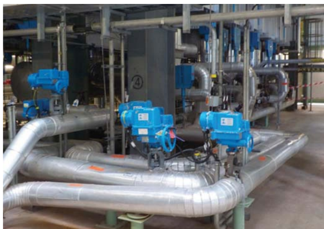
Blowdown valve installations at SSE Great Island prior to the upgrade.
