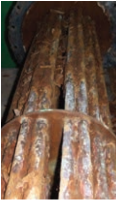
Scale on Heat Exchanger
