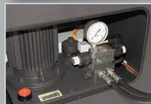
Dual-circuit hydraulic unit in cabinet base
