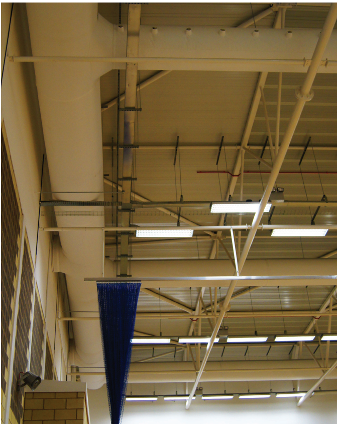
Plenum Distribution and branches all in Fabric showing Fabric Nozzles in the centre branch
