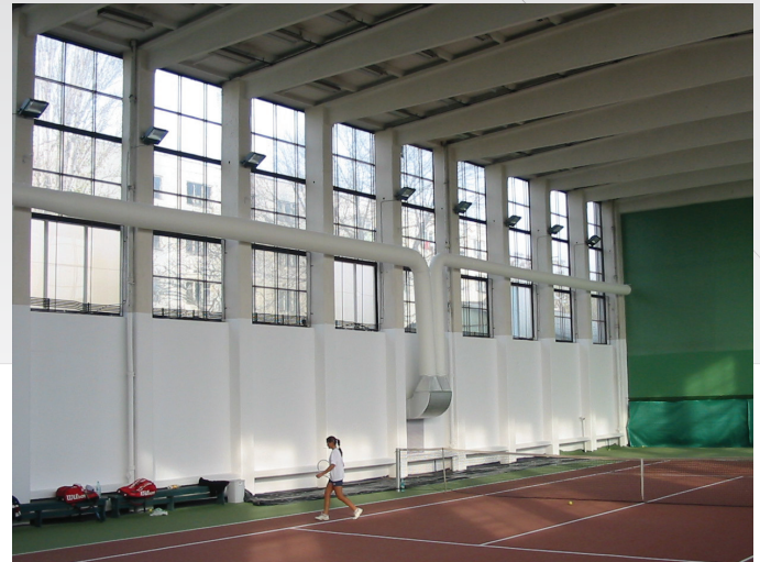
Fabric Ducting along the wall only - see why below...
