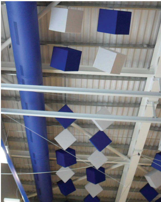
Whitmore School Sports Hall showing the different outlet diffuser style used along the walls to entrain more room air
