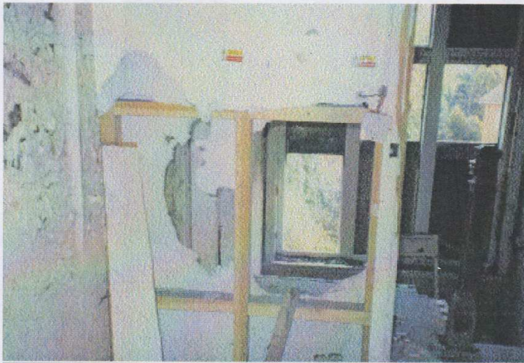
A severely damaged wall partition made of asbestos insulating board.
