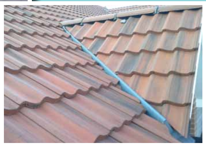
The completed installation: neat, tidy and effective – with minimal on-site time.
