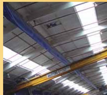
FILON practices what it preaches: rooflights in the FILON factory provide a pleasant and healthy working environment
