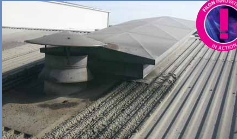
On this seven year old factory roof, the plastisol coated steel sheeting has failed due to exposure to fumes - but the adjacent Supasafe sheeting is 'good as new'!
