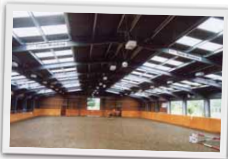
FILON took part in the 'Challenge Anneka' TV show in the eighties, providing rooflights for a riding centre
