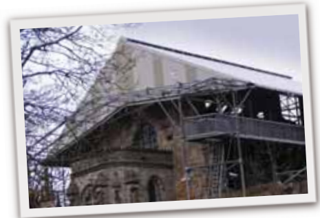
FILON rooflights provided daylight for restoration work at the Rosslyn Chapel, featured in Dan Brown's novel 'The DaVinci Code'
