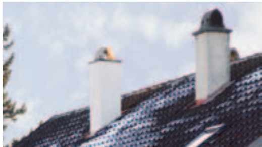
Costly heat is lost in the winter through a poorly-insulated roof. A sure sign of poor insulation is snow melting on a roof.
