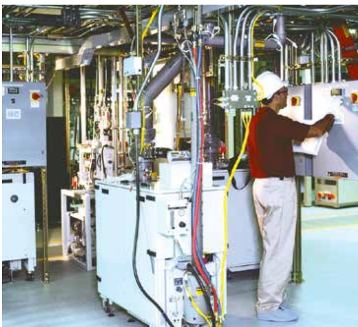
Heated forelines and pump exhaust lines in semiconductor subfab
