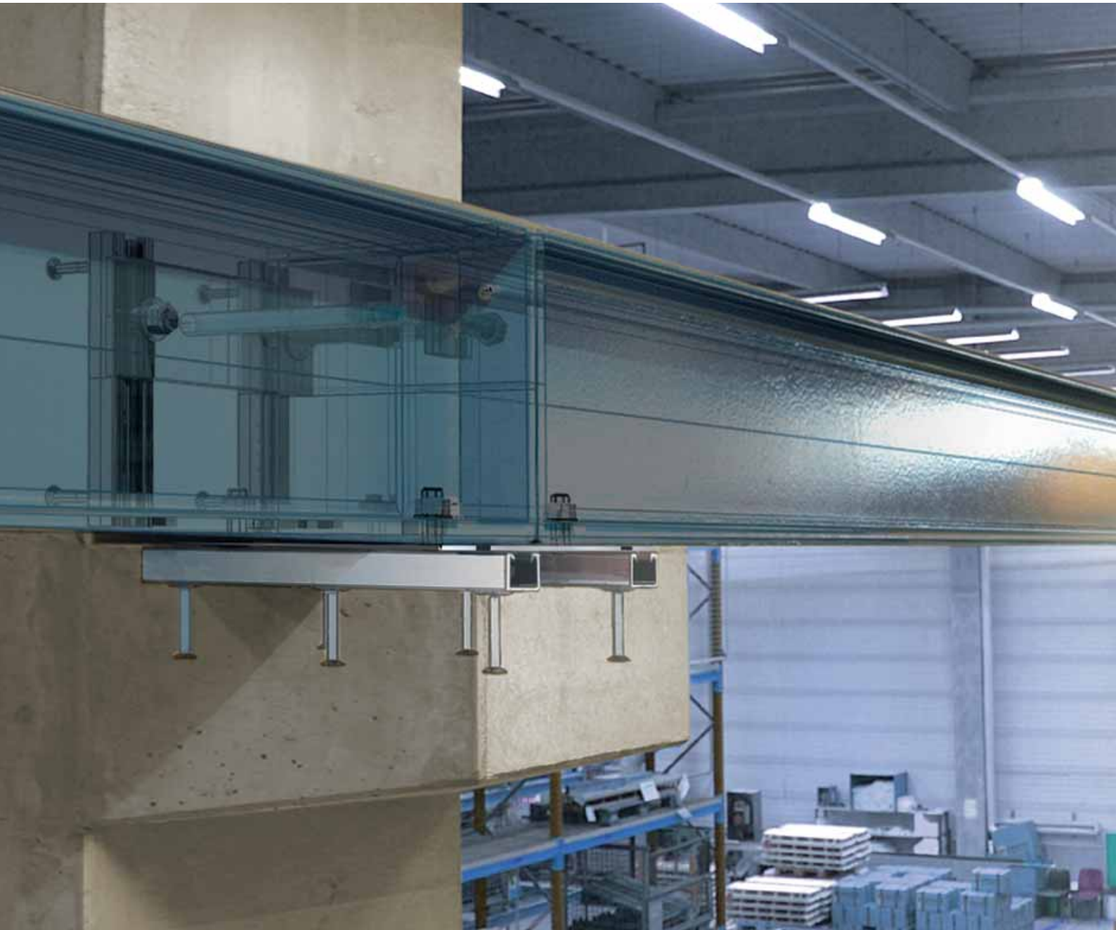
Overhead crane rail held in place with JORDAHL® T-bolts in anchor channels in a concrete corbel at a precast column
