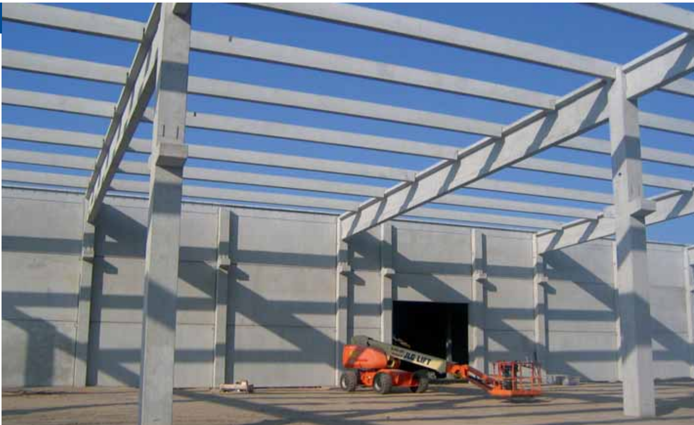
Structure of an industrial building completely preconfigured to be installed without any welding, drilling or concrete poured in situ.
