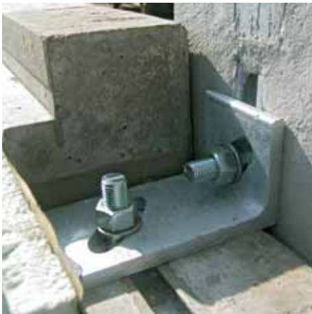
A pedestal wall connected to a support column using an angle bracket with diagonal slot holes
