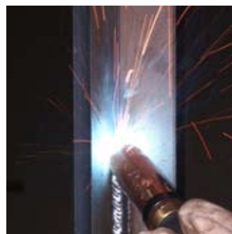
Conventional vertical weld xmas tree
