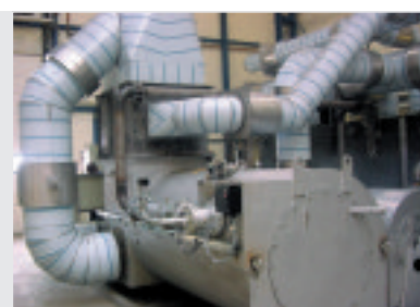
Afterburner with the heat exchanger →
