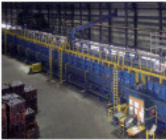
← Roller Hearth furnace line for annealing
