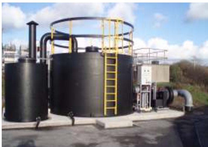
▲ Biotrickling filter installed for Dwr Cymru/Welsh Water
