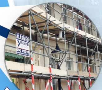
Construction Site And Scaffold Security
