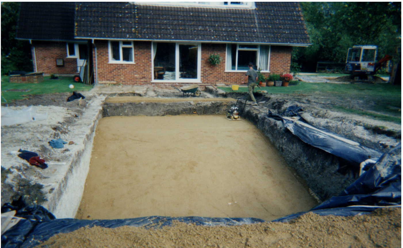
Lean mix 75mm base to shape. Well compacted. Main drain installed in deep end
