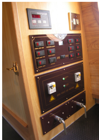
Well laid-out electrical control panels.
