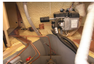
Webasto heater carefully installed in the coolest part of the engine room.
