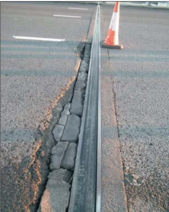
Incorrect joint selection - seal and rails rotating, pulling away grouts and fixings.
