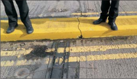
Joint going to nowhere . . . pavement cracking, bridge locking?
