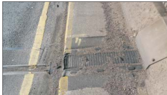
Joint not consistent, part single seal and part rubber - most likely to leak water from carriageway.
