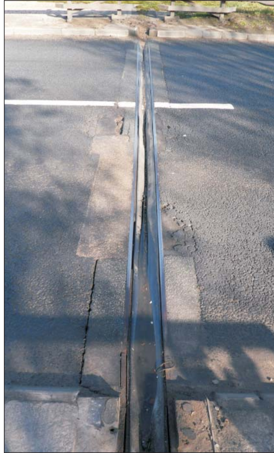
Cover plate missing at curb, seal in joint large and filling with debris. Poor installation of surfacing mounted edge rails leading to breakages.
