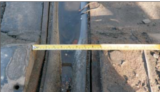
Width of joint does not accord with UK Highways Agency BD 33 - leading to short life and damage to fixity in road surface.
