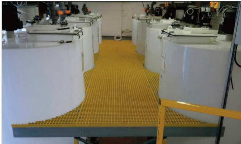
Tank Farm Platform
