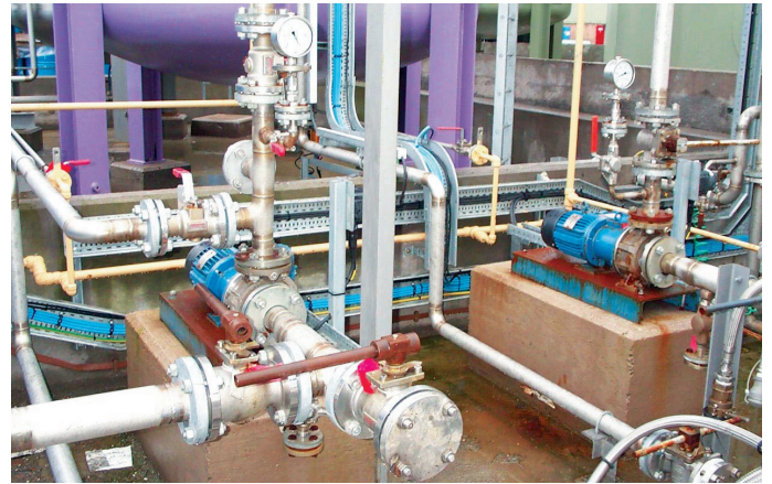
Verdermag Global pumps installed at a pharmaceutical production facility
