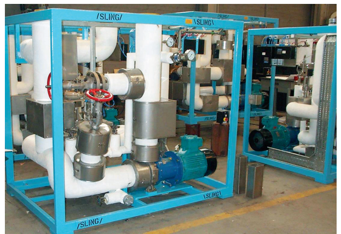
Verdermag Global pumps installed in cooling systems
