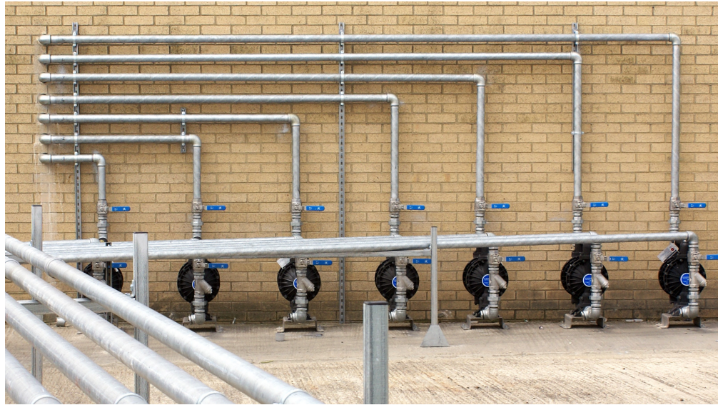
Above: A series of Verderair pumps designed and installed by Verder UK to moving solvent from silos to the process line.
