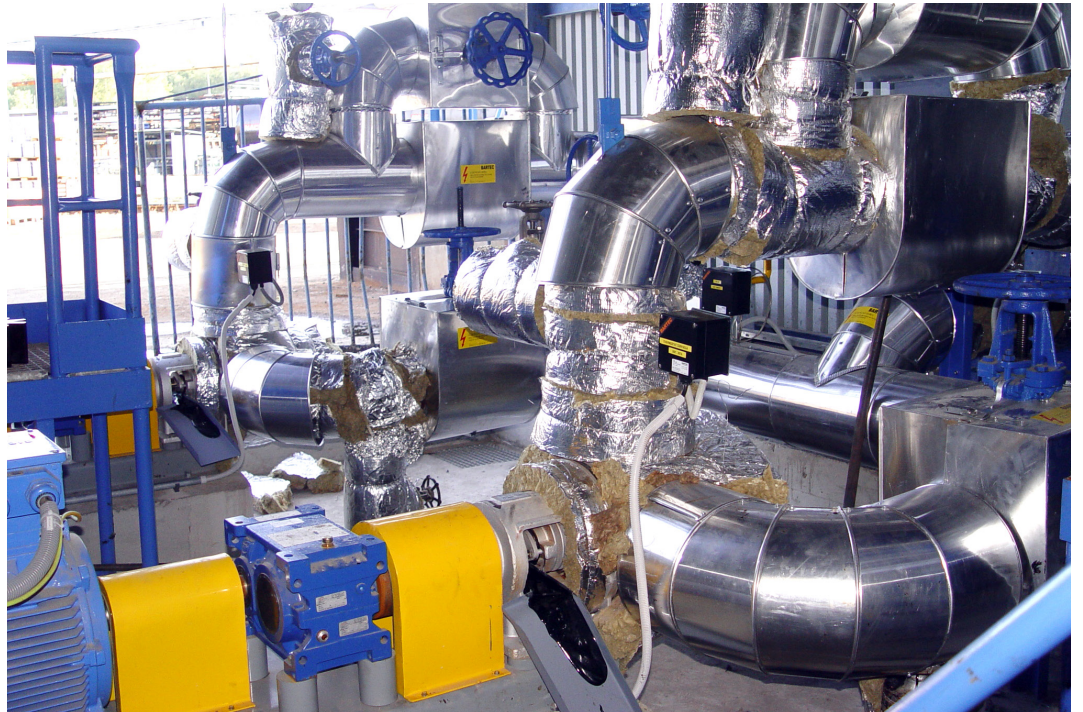
Verdergear pumps in a bitumen production plant
