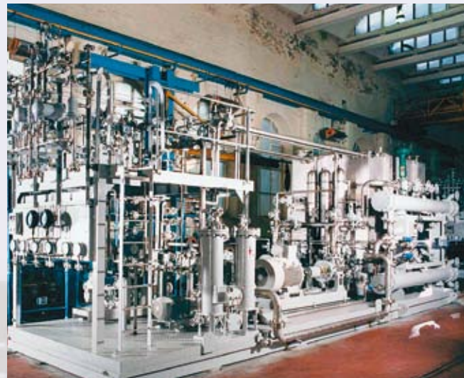
Compressed air cooling
