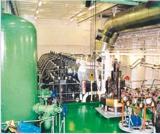
Ship engine cooling
