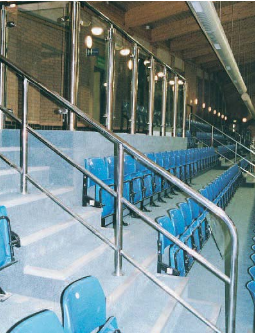
Triple rail barrier to spectator steps and disabled spectator balustrading complete with toughened glass infill panels.
