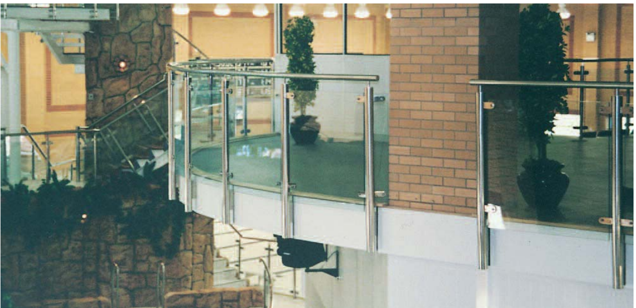
One of our projects. Curved stainless steel balustrading to viewing gallery complete with toughened glass infill panels.
