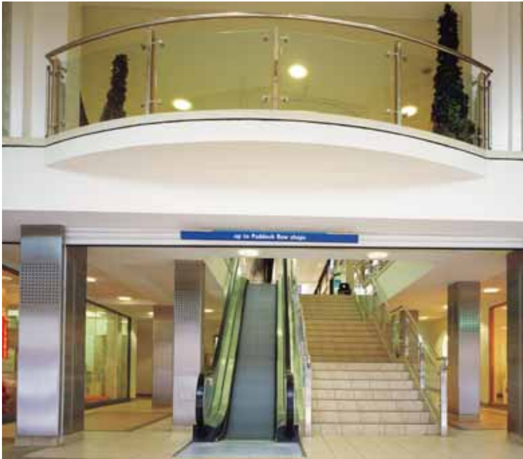
Stainless steel glass infilled balustrade to balcony edge.
