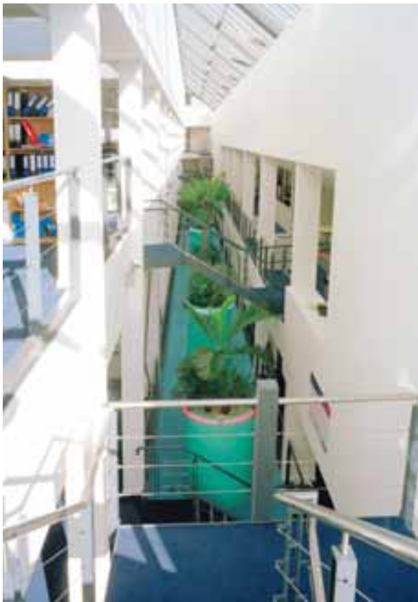
Powder coated mild steel balustrade complete with wire rope infill and stainless steel top rail, complement the atrium staircases.
