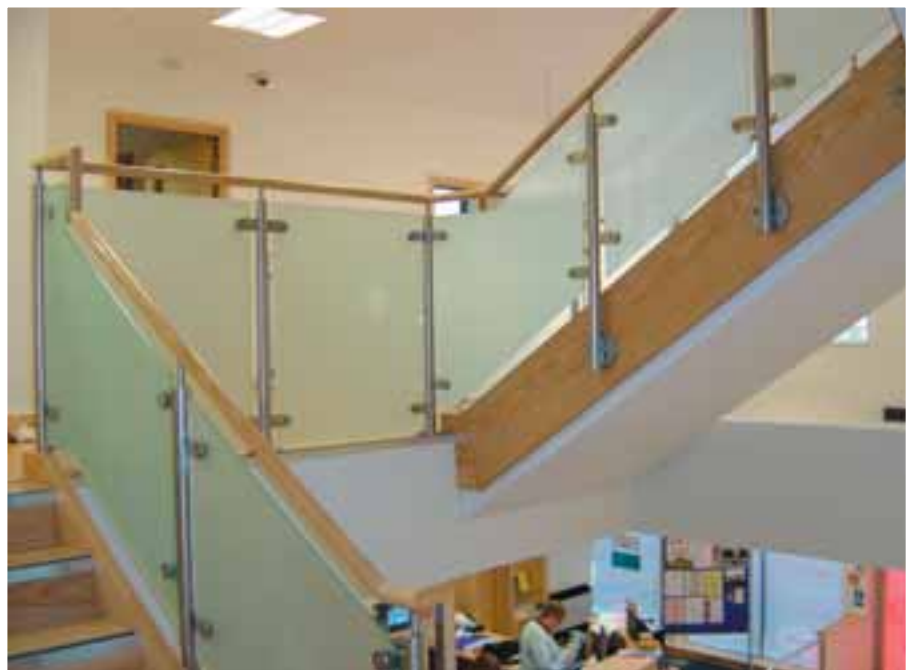
Stainless steel balusters with timber top rail and satinised glass infill.
