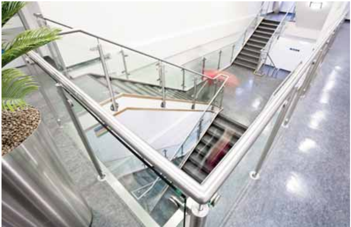
Complex six flight feature stairs complete with half landings – The Whittington Hospital London.
