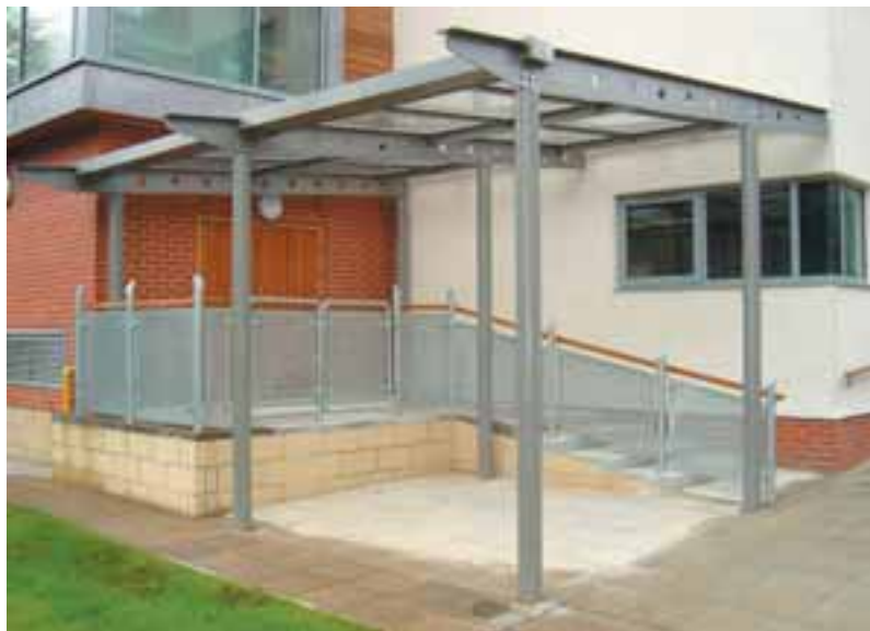
Canopy and galvanised external balustrading with a timber top rail and mesh infill panels.
