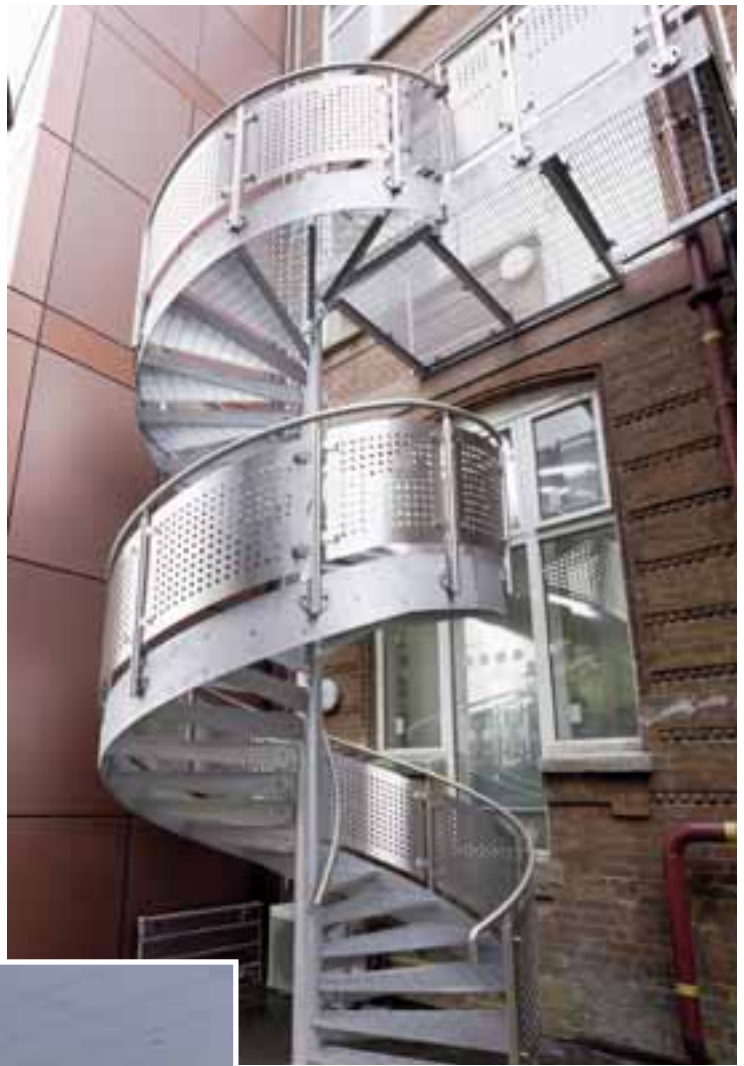
External mild steel spiral fire escape stair with perforated aluminium panel infills.
