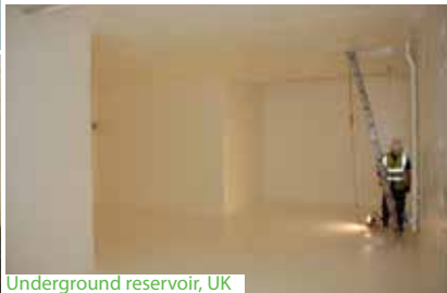
Underground reservoir, UK
