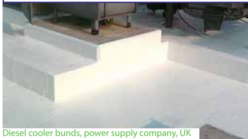
Diesel cooler bunds, power supply company, UK
