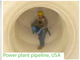
Power plant pipeline, USA
