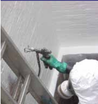
Wet well, pumping station, UK
