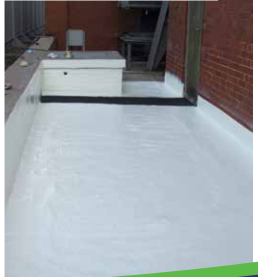
Diesel cooler bund, major power supply company, UK
