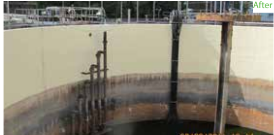
Digester, UK water treatment works
