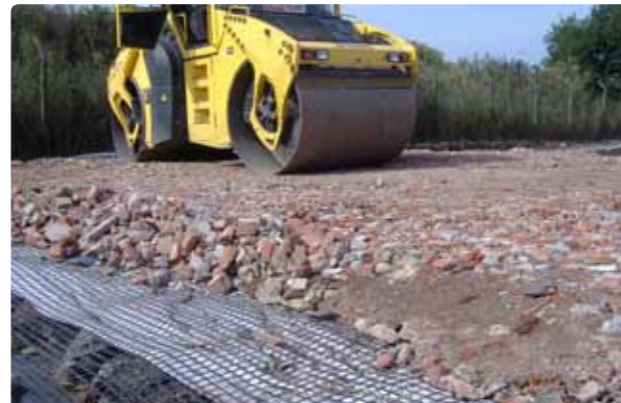
Abweb beneath crushed hardcore in plant yard
