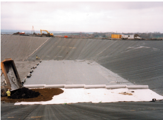
Long view of site with Pozidrain rolls clearly visible in the foreground
