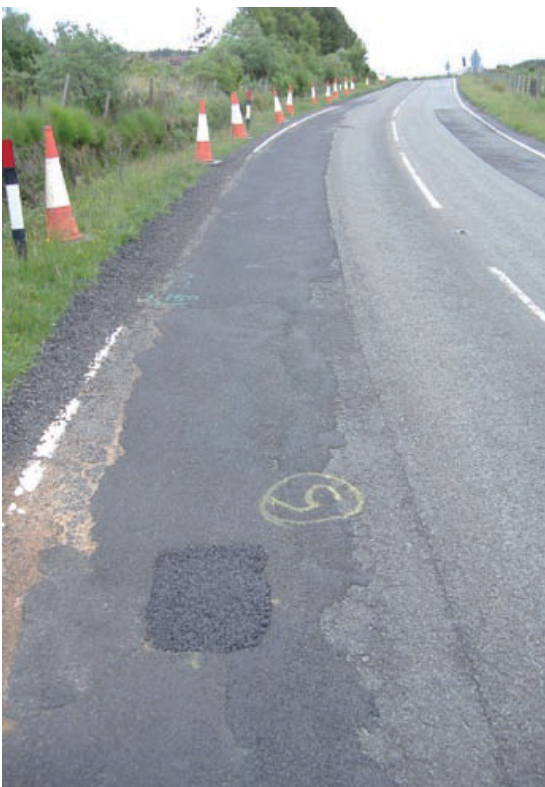
Example of verge failure with evidence of previous repairs
