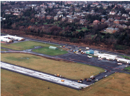
Aerial shot of installation. White areas show Rotaflex prior to being overlaid with asphalt
