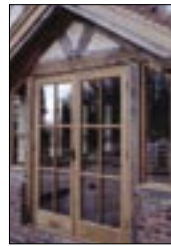
EFRo3: External fully glazed oak patio doors.
