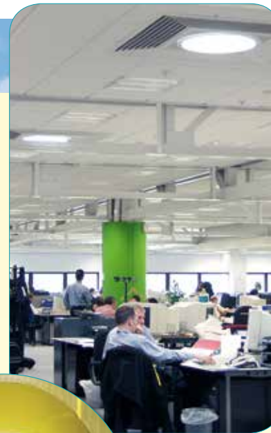
SUNCATCHER installations at the BMW head offices
