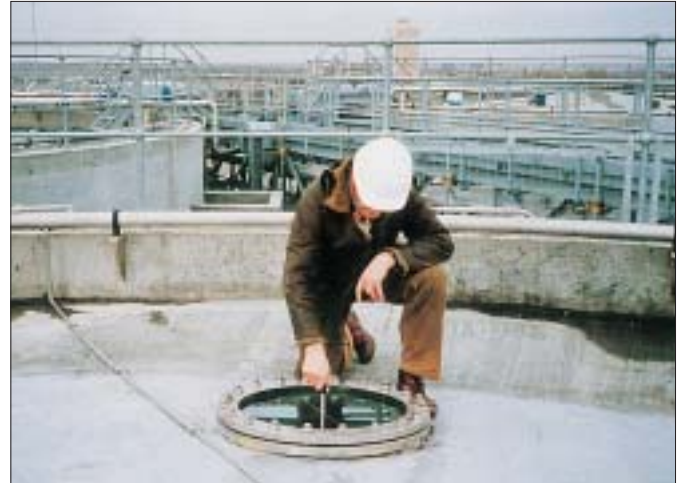
Sight port and Wiper on water treatment plant.
