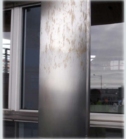
This column showed signs of corrosion shortly after installation. The lower area has been treated with Cleaner 61.
