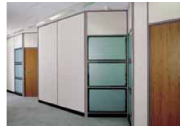
135° posts to create a faceted corridor with solid and transom glazed partitioning
