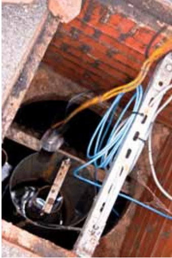
A manhole cover removed and an interceptor being checked for oil content prior to cleaning.
